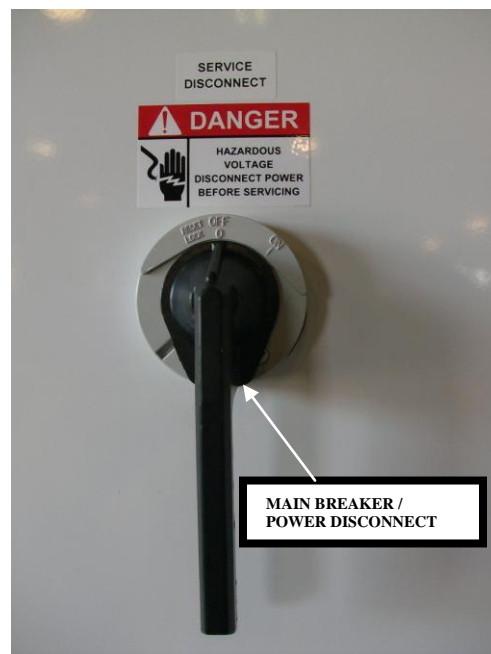
MAIN POWER DISCONNECT MAIN POWER CABINET PHOTO #3
